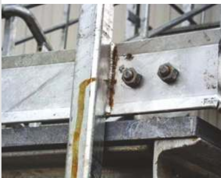
Bleeding and weeping welds
